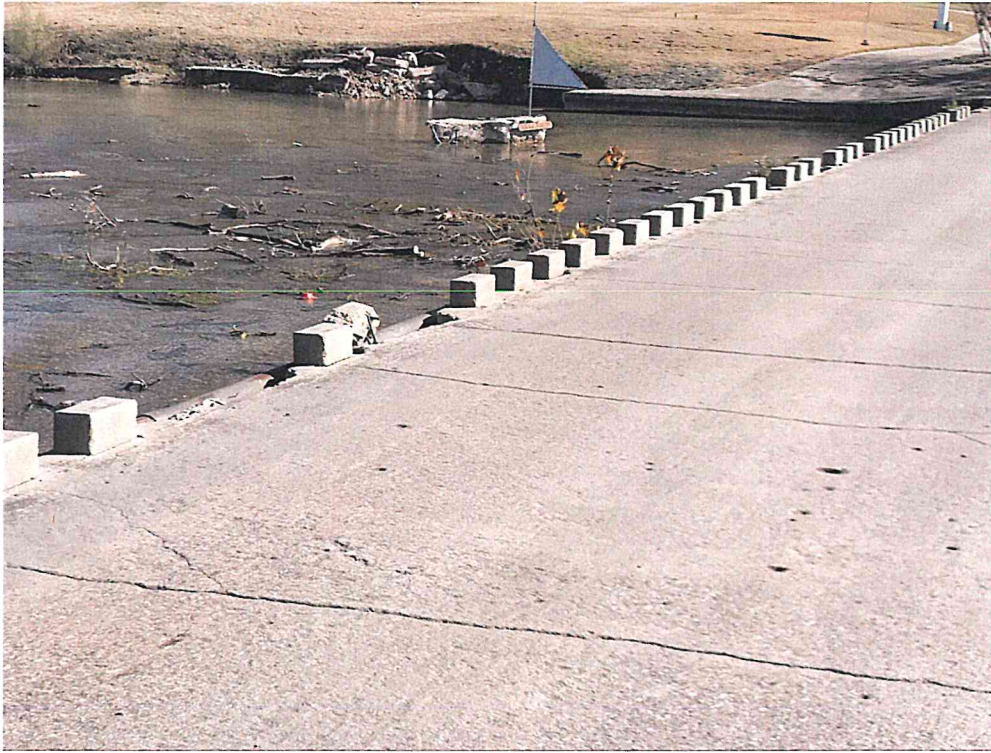
Figure 5 – Missing “Teeth” of Sawtooth Curb Looking Back to the East
