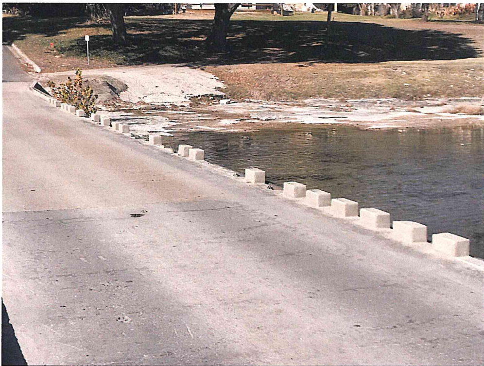
Figure 4 – Missing “Teeth” of Sawtooth Curb Near Northwest End of Crossing
