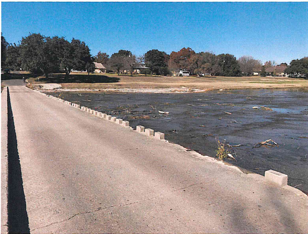
Figure 2 – Missing "Teeth" of Sawtooth Curb
