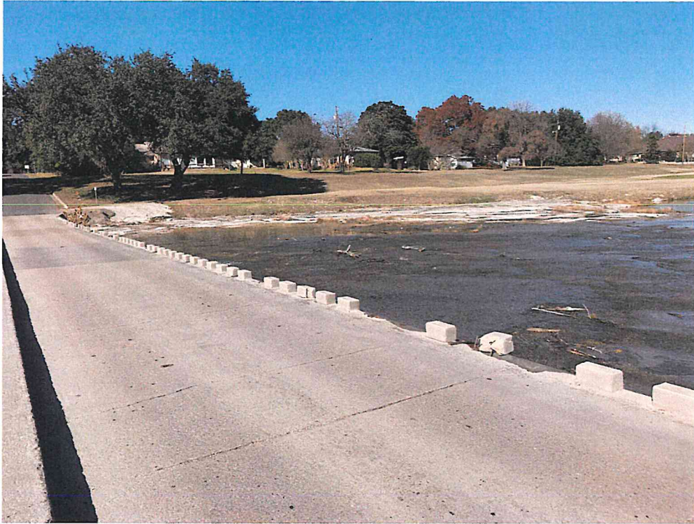
Figure 3 – Missing “Teeth” of Sawtooth Curb
